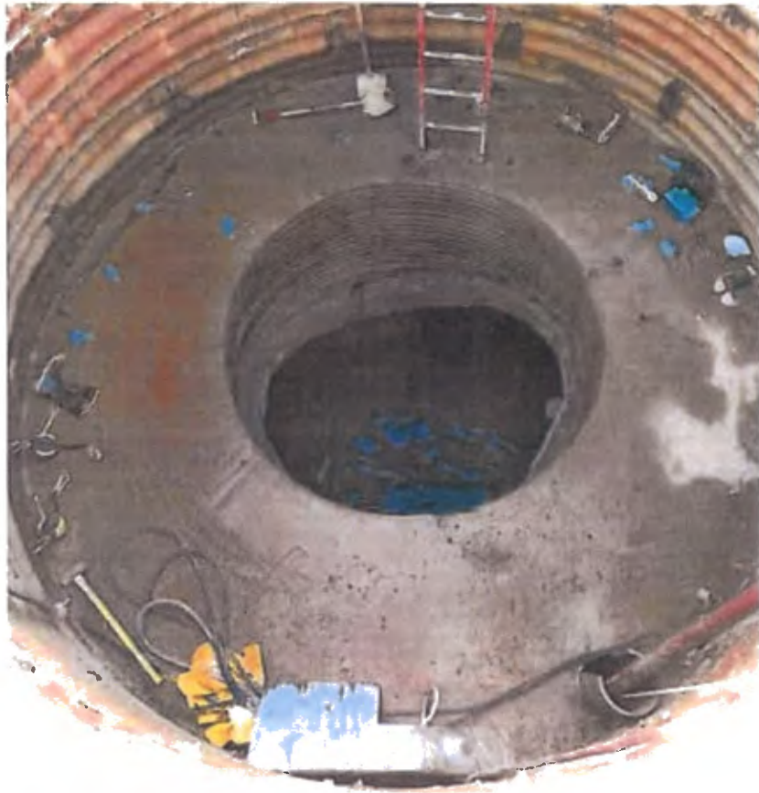
As part of the Segment 4 repairs, a suite of trenchless methods were used, including CIPP, cementitious Centripipe and grout-in-place liners.
